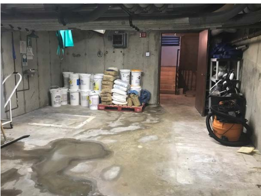
The Banyan pump room cleaned & organized by engineering.
