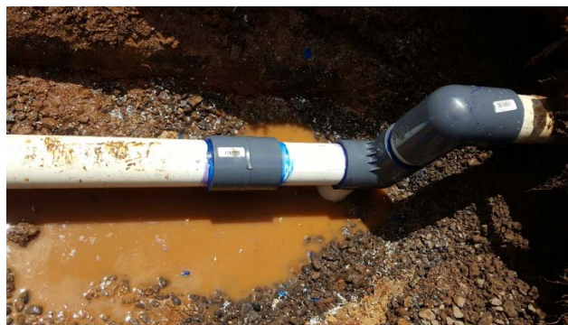
Landscaping with Engineering helped repair a main water line break fronting unit 3113. Forty five degree Elbow cracked
