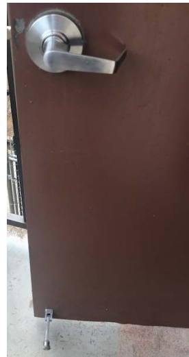
Engineering replaced the door handles and door stops of the garage exit doors.
