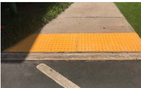
Engineering replaced the yellow matt at the entrance to the Alii east wing.
