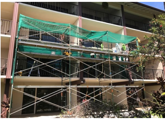
JD Painting started and completed spalling on units 3104, 3204 & 3205. Unit 3204 had some major damage to the lanai.
