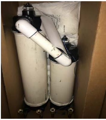
Oahu Air Conditioning replaced the Heat exchange for the Banyan Spa, which was under warranty.
