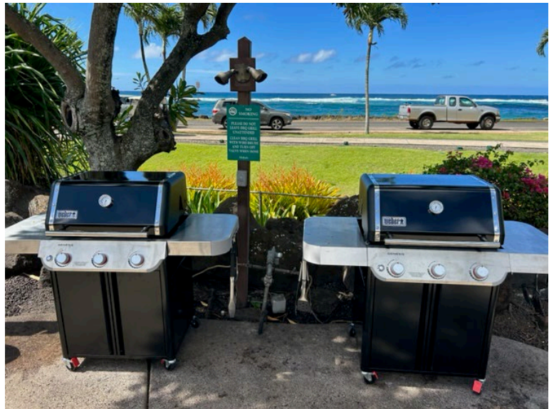
Engineering started the replacement of the BBQ grills, starting with the Banyan pool. All grills will be changed out within the next month.
