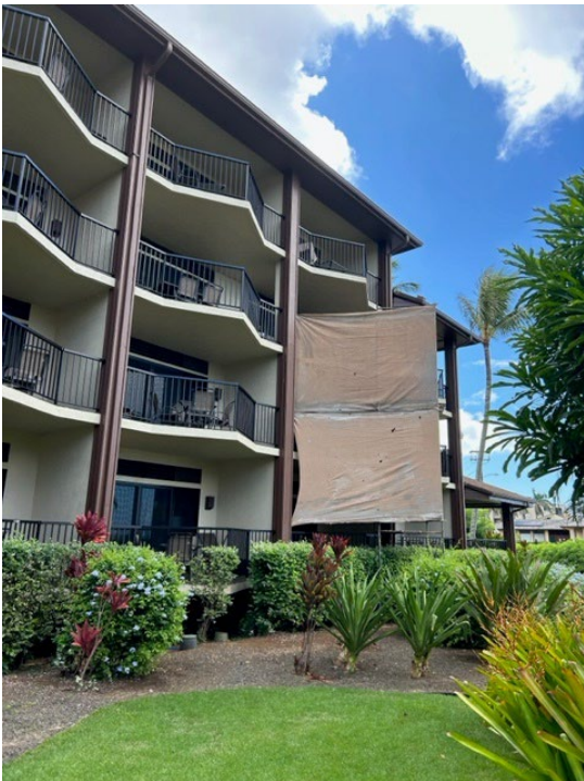
JD Painting completed the spalling of unit 2302 and started unit 2402 as we found a crack in the lanai.
